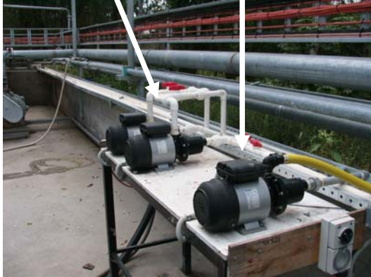
Figure 2.7: SBR feed pumps and prefermenter feed pump.
