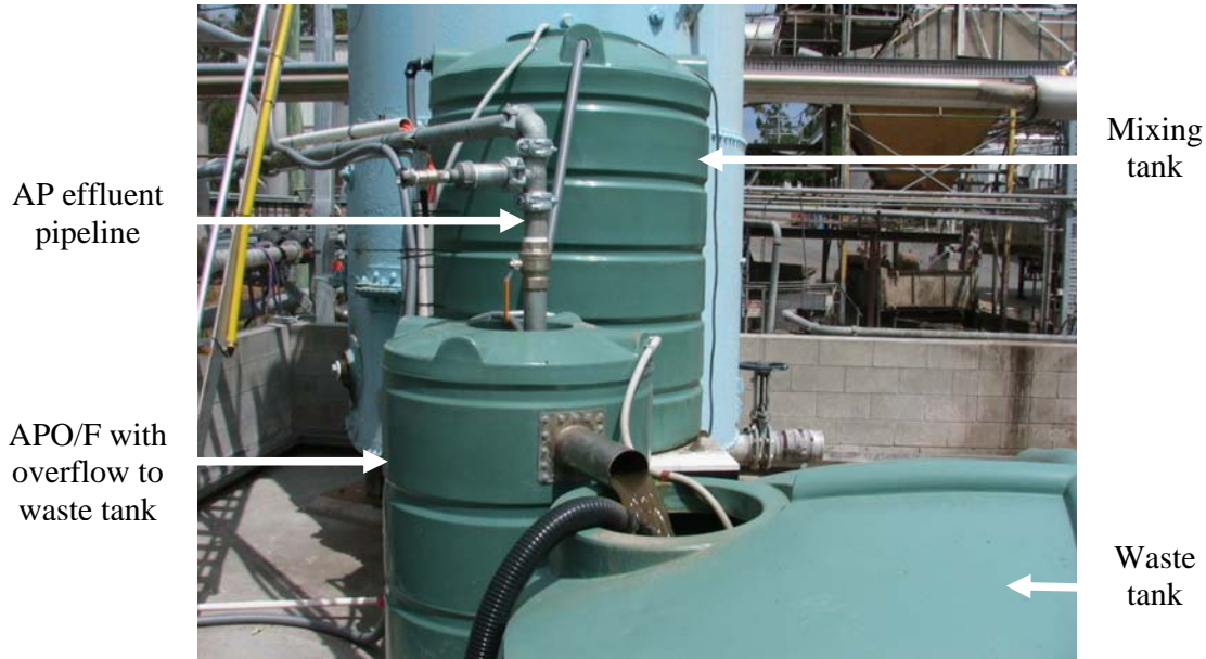
Figure 2.5: Anaerobic pond overflow tank, mixing tank and waste tank.
