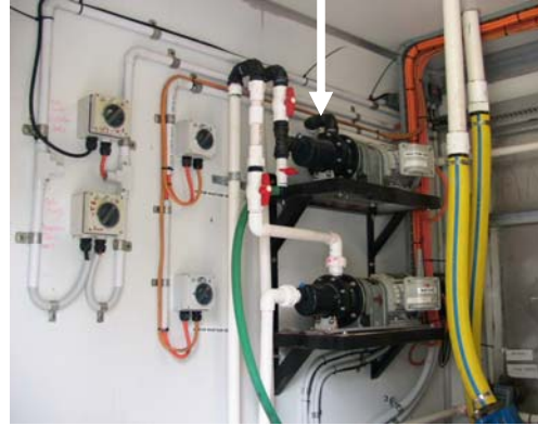
Figure 2.8: Location of WAS pumps in hut.
