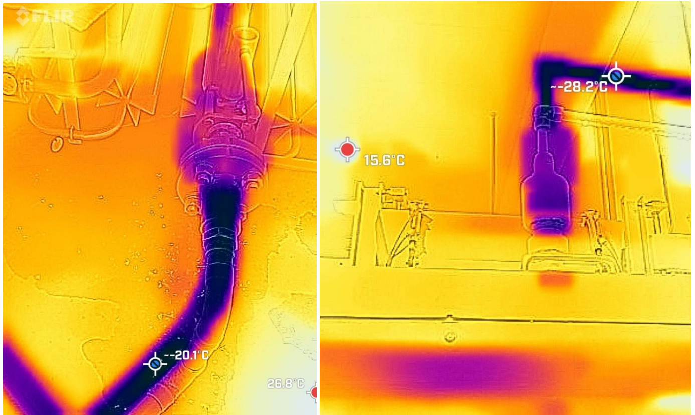
Figure 5: Evidence of the requirement for lagging on LCO2 from storage tanks (left) and LCO2 line within the boning room (right).
