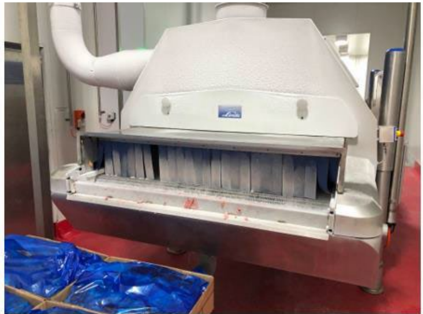
Fig 4 cooling tunnel in operation test phase
