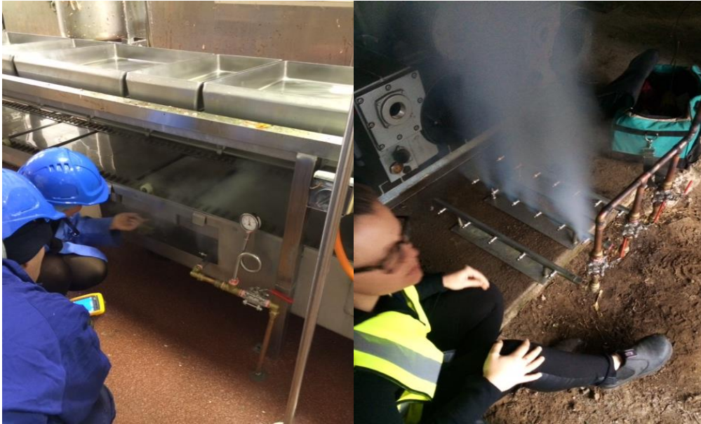
Figure 13. Steam bar attached to sanitation point on table | Figure 14. Steam bars connected to boiler under plant floor.
