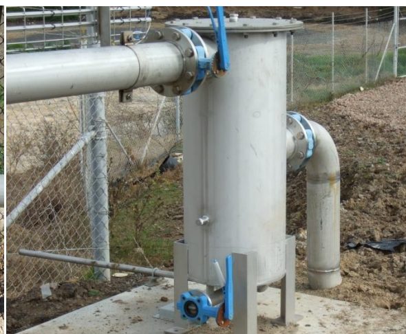
Photo 6: Knockout pot in biogas train.
