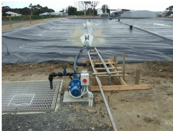
Photo 4: Typical stormwater removal system.
