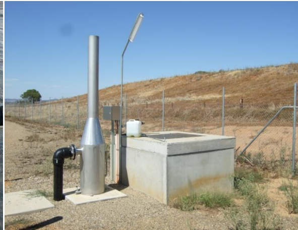
Photo 3: Hydrostatic release valves.
