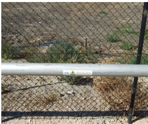
Photo 5: Above ground stainless steel biogas pipe.
