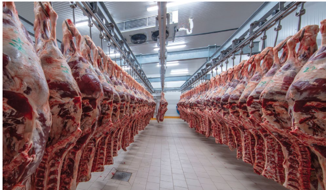
Refrigeration area in a meat processing plant
